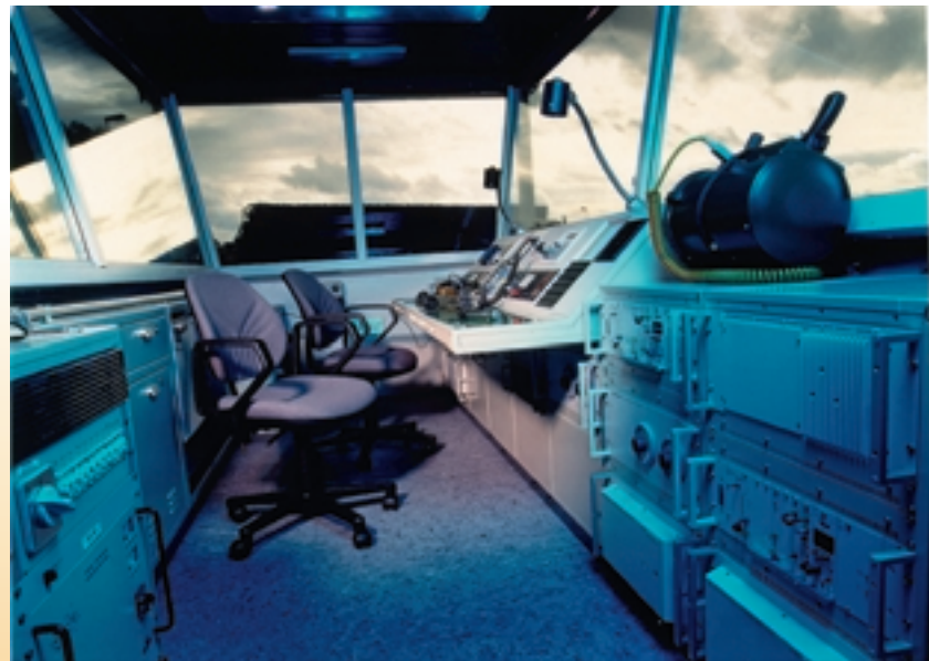
FIG 5 Control tower cabin with three ATC workstations
